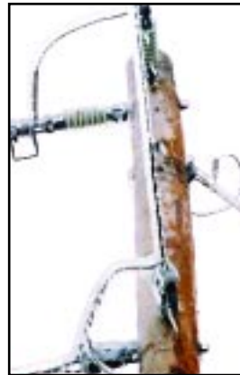
A heavy coating of ice on poles and electric equipment made repair work a treacherous and time-consuming affair.
