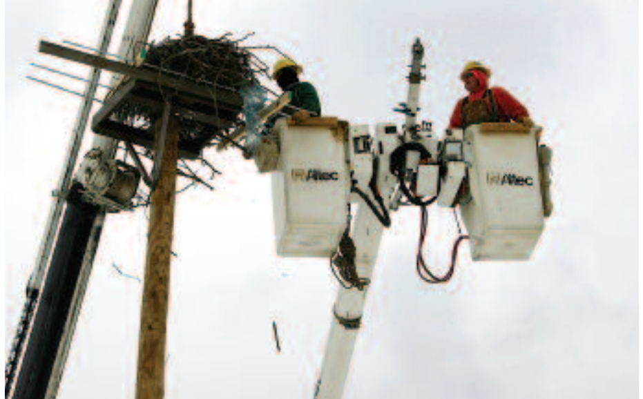
Tri-County line workers Don Williammee, left, and Rocky Wiedman guide the osprey nest to its new perch on the Cowanesque Valley High School grounds.
