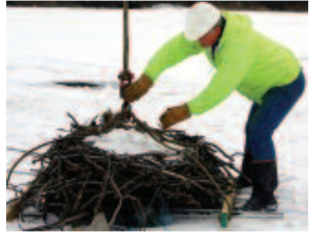
Westfield crew chief George Harer repositions an osprey nest before its transfer to a nesting platform on top of a utility pole outside of Cowanesque Valley High School.
