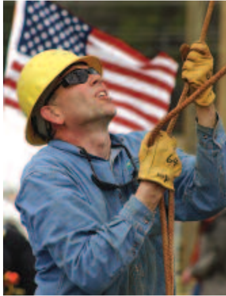
Bob Mathers, serving as the Tri-County crew's ground man, hoists a transformer up the pole to teammates Dave Gibson and Jim Succowich during the transformer change-out competition. The co-op posted one of the best scores in the rodeo for this event.
