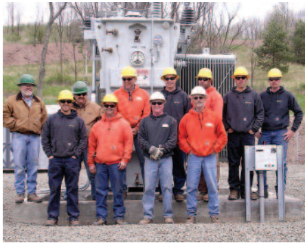
POWERING UP: Members of Tri-County's operations and engineering departments stand in front of the new 5-megavolt-ampere transformer at the Sullivan Substation near Mainesburg after the rebuilt substation was energized and put into service April 30. Pictured are Mark Whitney, Joe Mickey, Ron Hager, Chris Payne, Bob Mathers, Dave Gibson, Eric McRoberts, Ron Sawyer, John DeWitt, Brian White and Steve Brewster.
