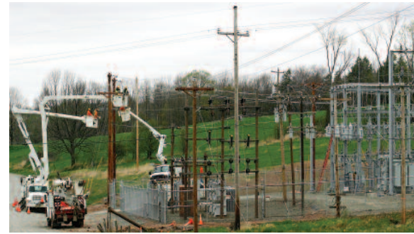
SUBSTATION TRANSFORMATION: Tri-County line crews work to tie in the rebuilt Sullivan Substation with the cooperative's distribution system on Thursday, April 30. The changeover from the old portion of the substation to the new (steel structure on right side of photo) required a 3.5-hour planned outage and a well-coordinated effort involving about dozen co-op lineworkers and technicians.
