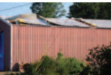
A microburst tore the overhead garage door from Tri-County's Liberty District building and blew off a 40-foot section of sheet-metal roofing on the south side of the structure on June 10.
